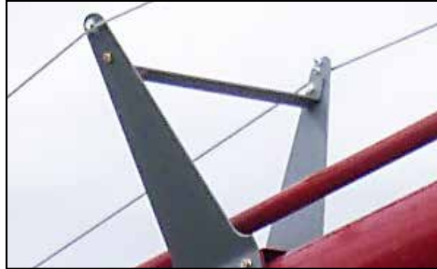
Fig 44 - Cable clamps on truss risers
